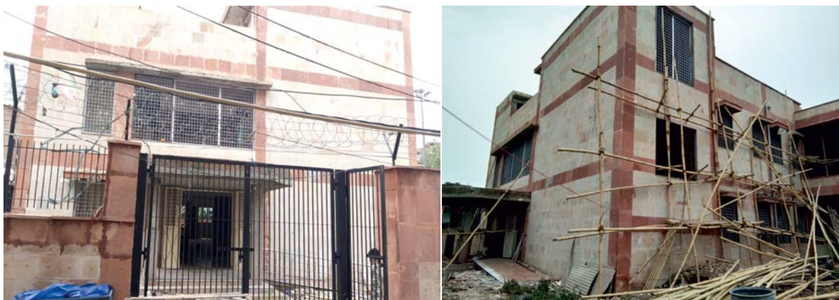
Community Facility Center (Choupal) at D-block, New Seemapuri (under construction) Out of funds from Trans Yamuna Area Development Board
